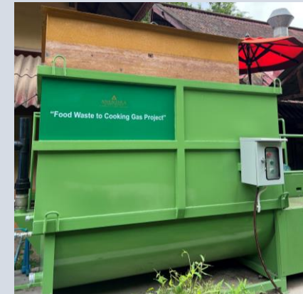
Biogas digester at Anantara Golden Triangle
